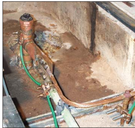
Figure 2. The DPTE’s primary grounding electrode, upper left, near the center of the subbasement. The chemical-type copper electrode is surrounded by bentonite for improved earth contact. Ground resistance is checked every six months and ranges between 3.0 ohms and 3.5 ohms. The 750-kcmil tinned-copper grounding electrode conductor, foreground, is bonded to
