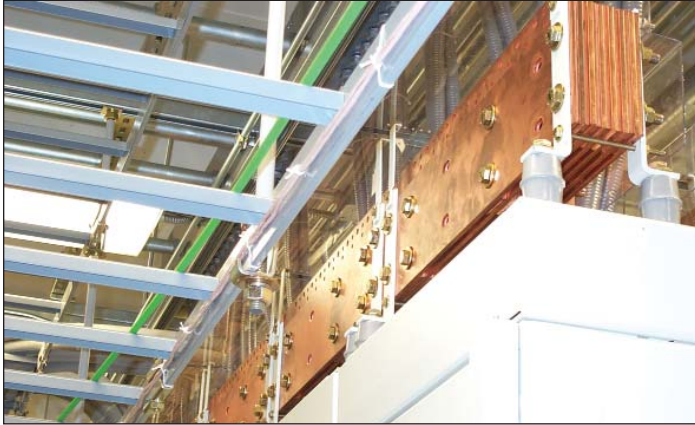
Figure 1. Electrical systems in Internet data centers are designed to accommodate higher power densities than those in conventional office space. The robust power buses shown here seem more appropriate for heavy machinery than for racks of electronic equipment. Power usage in IDCs has not been as high as originally anticipated, but power quality requirements remain more stringent than those of almost any other industry.
