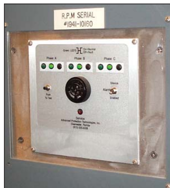
Figure 10. A system provided by Reliable Power Meters (RPM) continuously monitors and logs such power quality parameters as voltage, current and waveform.
