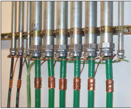
Figure 8. In most instances, large grounding conductors at the DPTE are not encased in conduit, but one tenant elected to do so in its system. The IEEE-recommended practice for this installation calls for bonding the conductor to the conduit at both entrance and exit points.
