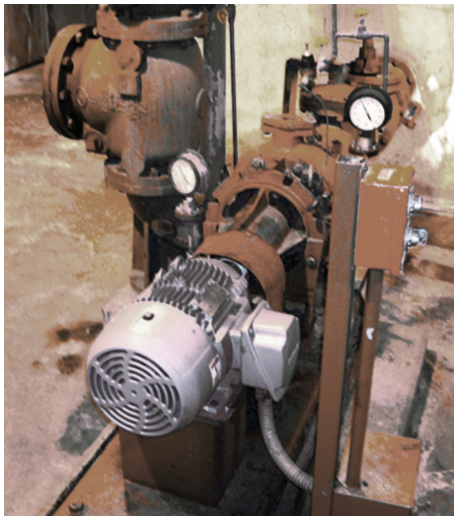
A new, 10-hp Siemens copper-rotor motor installed on an excess activated sludge pump at the ACSD Menands plant. Not shown in the photo is the variable frequency drive, that, when used to control the motor's speed and the pump's throughput, resulted in significant energy savings. Payback for the motor-VFD combination was well less than one year.
