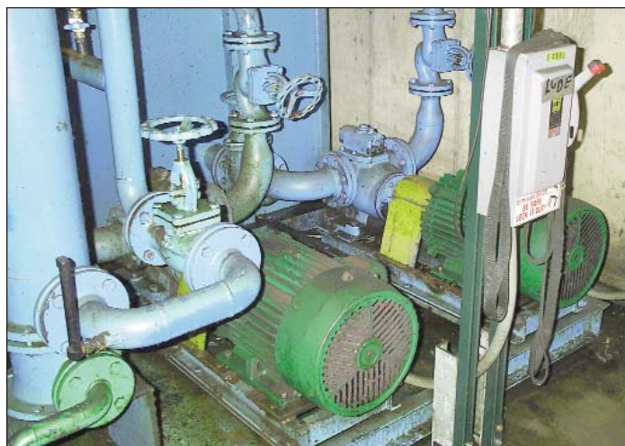
Figure 2: Two 100-hp NEMA Premium motors drive lubricant pumps on one of OCP's rolling mills. Operating at 95.0% efficiency (75% of full load) the Toshiba EQP III motors save the company 16,700 kWh per year each. Payback of the cost of the new motors compared with rebuilding existing standard-efficiency motors was less than two years. In addition, each motor reduces carbon dioxide emissions by almost 11 tons annually.
