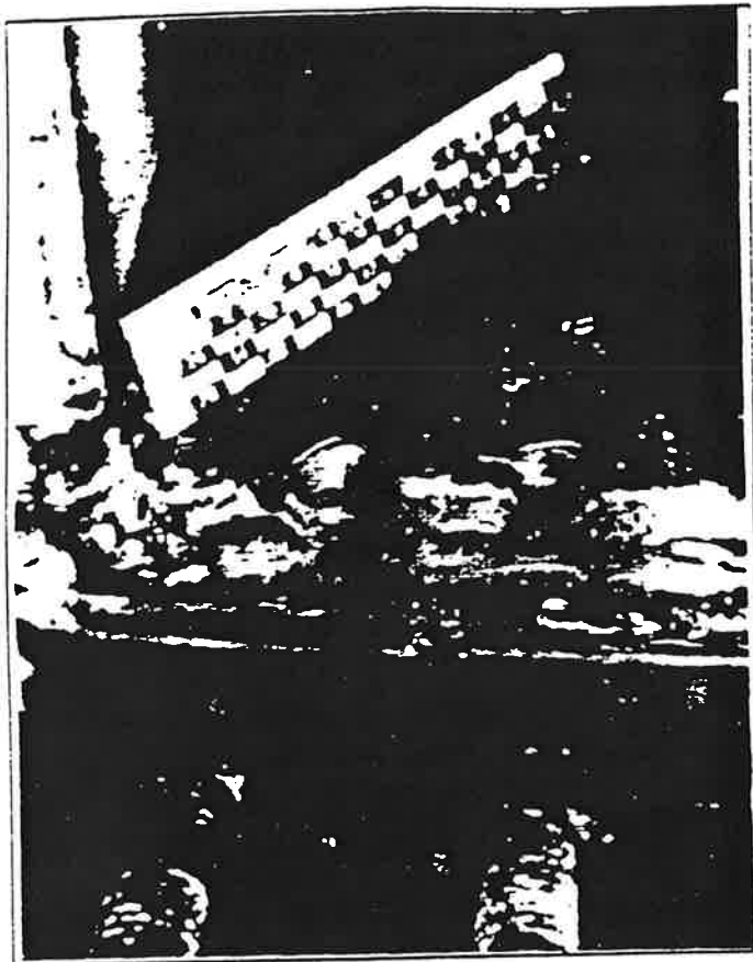
FIGURE 9 Corrosion of coated steel waterbox resulting from pinhole failure of coating.
