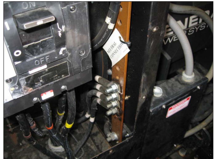
Figure 4. The neutral-ground connection (bottom center) at the emergency generator constitutes a short condition because the transfer switch is three-pole, meaning that the generator is not a separately derived source. The improper connection can inject current into the grounding system.
