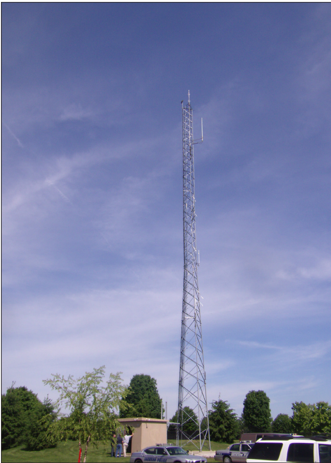
Figure 1. Jackson Township's fire and police communications equipment is housed in the small remote communications building to the left of the 140-ft antenna tower. The tower has attracted many lightning strikes, and because it was poorly grounded, lightning energy was able to damage equipment in the building and elsewhere on the municipal campus.
