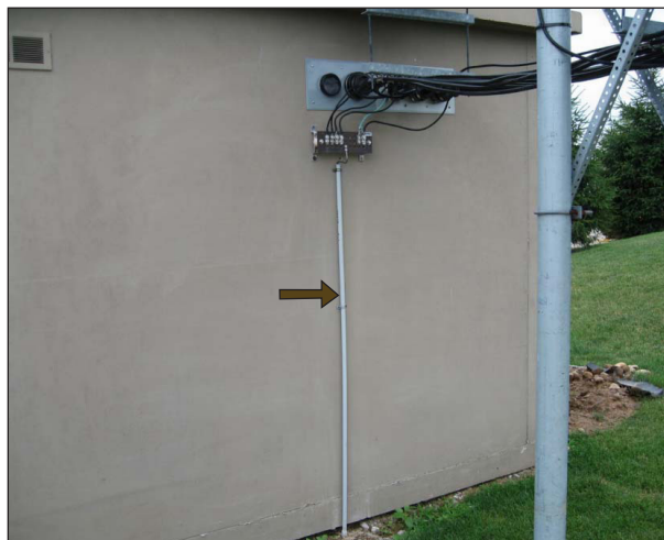
Figure 8. A separate earth connection at the tower/transmitter site was made from the outdoor grounding bar seen just beneath the wall penetration. The grounding conductor (in conduit, arrow) connects with the tower ground at the opposite side of the building, forming a three-way ground loop.
