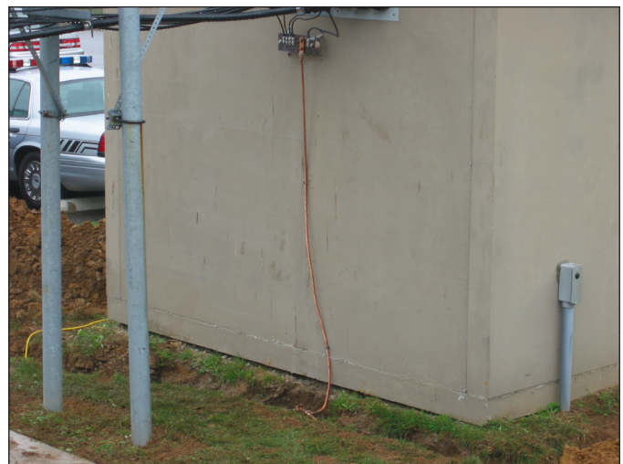
Figure 13. A new AWG 4/0 copper ground connector bonds the outdoor ground bar to the ring using an exothermic weld and an approved UL 467 compression terminal.
