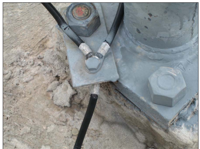
Figure 7. One of three existing earth connections at the antenna tower was made to a tower leg (upper photo). It terminated at an 8-ft grounding electrode. The mechanical connection to the tower (lower photo), was made to a galvanized and painted steel tab, which was itself bolted to the galvanized steel tower support flange. This connection method imparts high resistance and is not recommended.
