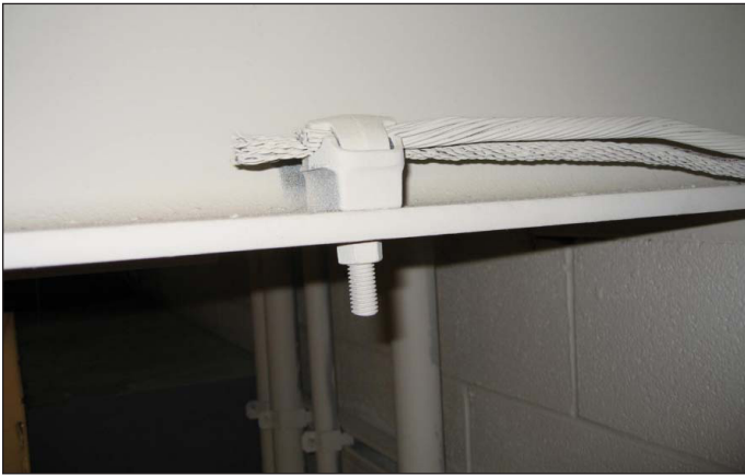
Figure 5. A building steel grounding conductor and a braided lightning rod (air terminal) down-conductor are shown connected to a painted steel member by an unapproved bar-tap. Building steel connection to earth was unknown and the connection has high resistance. The air terminals should have been earthed to the grounding electrode system or ring ground outside the building.
