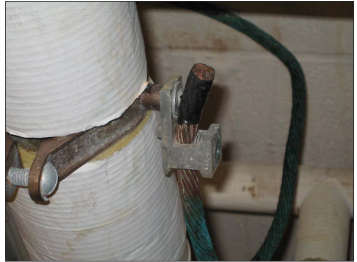
Figure 3. An improper grounding connection between two flanges on the street side of the water line. Flanges were also missing jumpers to provide a path to earth.
