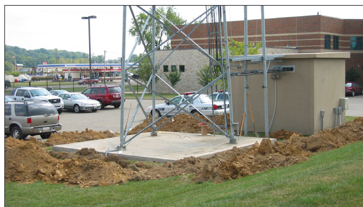
Figure 10. A new 3-ft deep trench surrounding the tower and remote communications building contains an AWG 4/0 bare copper ring ground, three new electrodes and connections to the tower, two existing electrodes and the building's electrical system ground.
