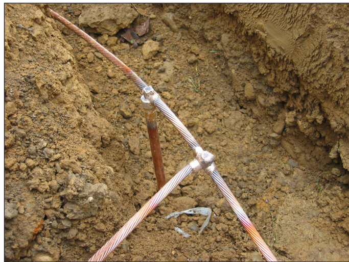
Figure 12. Exothermic welds connect new electrodes with the copper ring ground. A conductor from one of the tower legs is seen at lower left.
