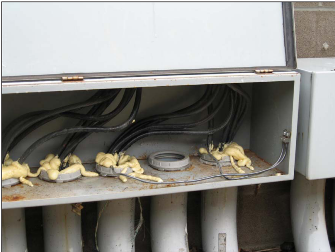
Figure 2. A pair of grounding conductors (front right) improperly connected to a utility meter cabinet. The cables ran 100 ft to the main wireway inside the safety center, and their length invited stray current pick-up by the grounding system.
