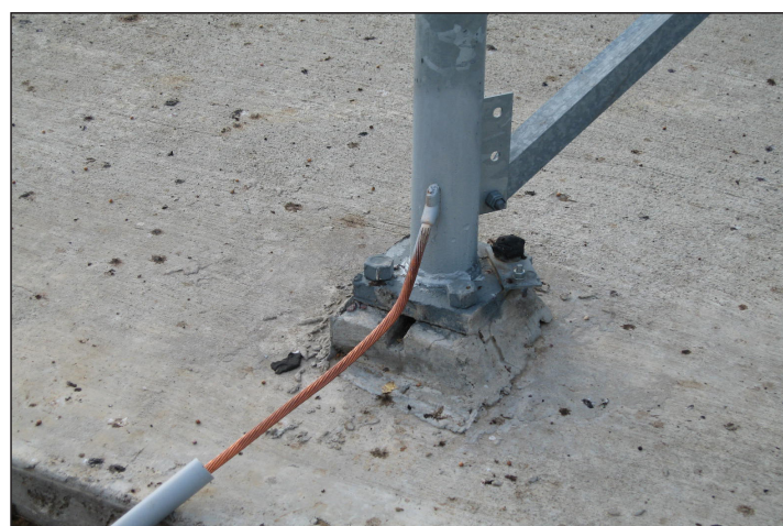
Figure 11. An exothermic weld bonds a grounding conductor to a tower leg. Zinc galvanize was removed from the leg prior to making the weld. Protective paint covers the new joint area.
