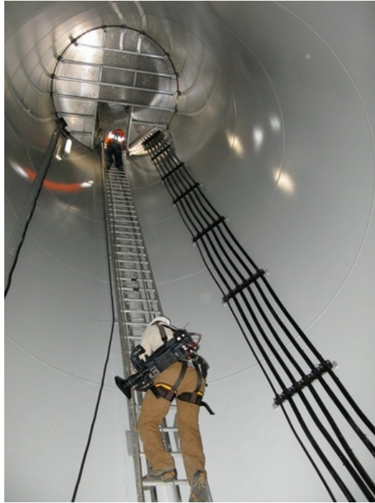
Figure 1.1 Heavy gauge copper cables within the wind turbine tower
