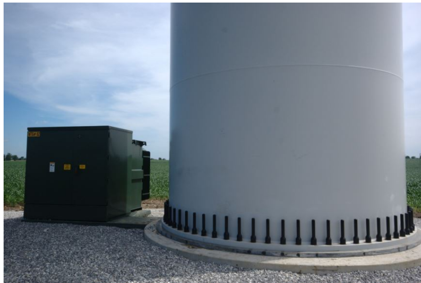
Figure 1.2 Step-up transformer located on the wind tower pad
